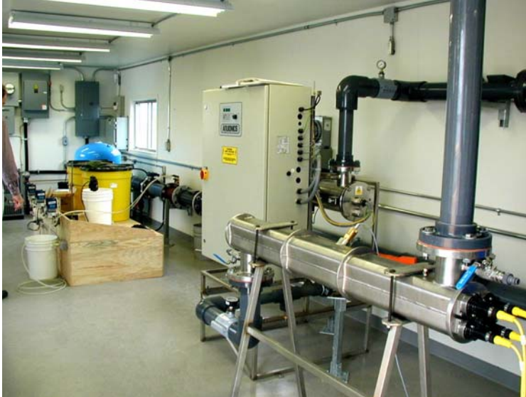
UV reactors disinfect water in the City of Winnipeg UV pilot testing facility (Photo: City of Winnipeg/Duane Griffin).
